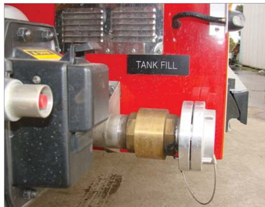
Figure 15 – water tank fill point
